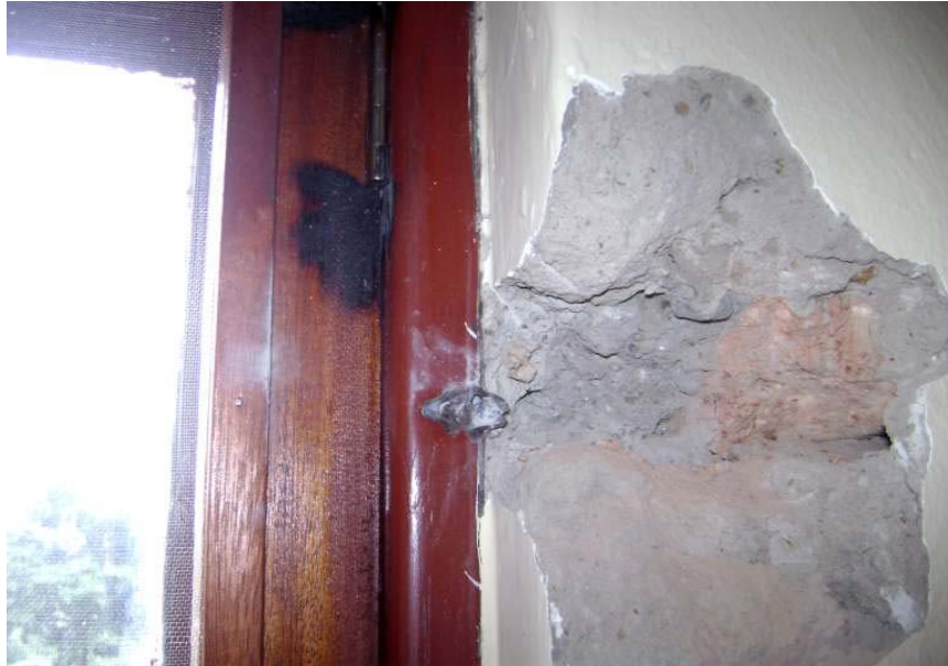
Figure 2 . The bullet hit the metallic window and lodged into the wall.
